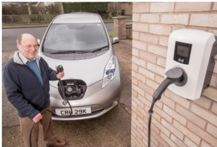
Level -1 Charging (EVSE)
